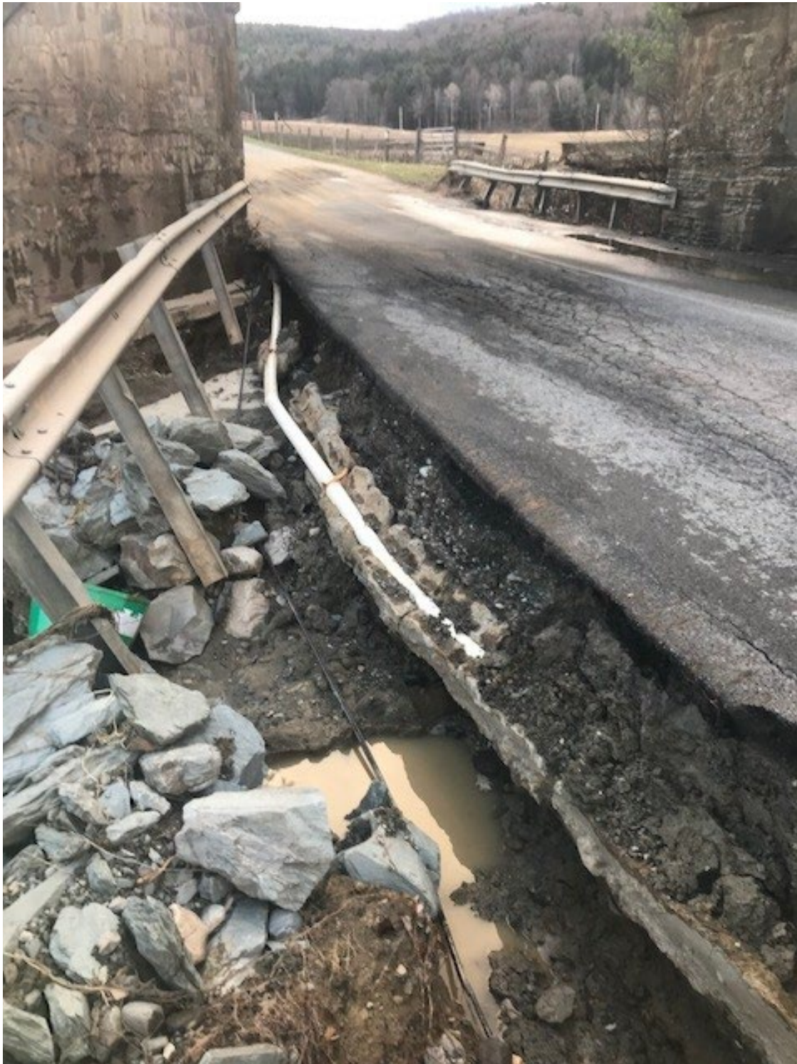
South Street Trestle Bridge Washout – April 2019
