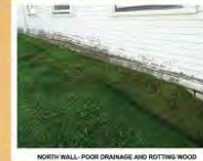
NORTH WALL- POOR DRAINAGE AND ROTTING WOOD
